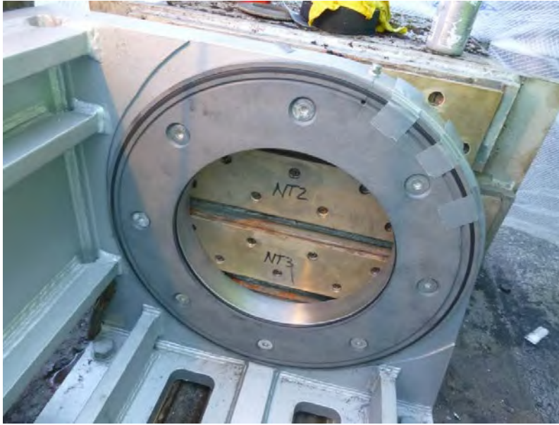
Figure 12-26. Spillway Tainter Gate Trunnion Thrust Washer.
