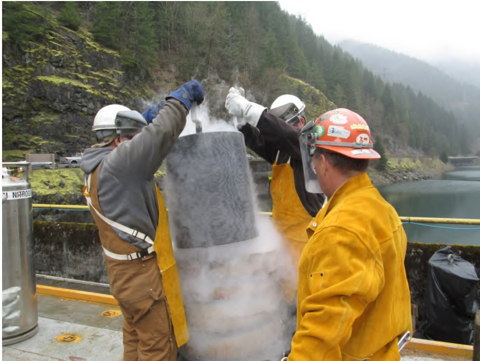
Figure 12-24. Spillway Tainter Gate Trunnion Bushing Freeze Fitting.
