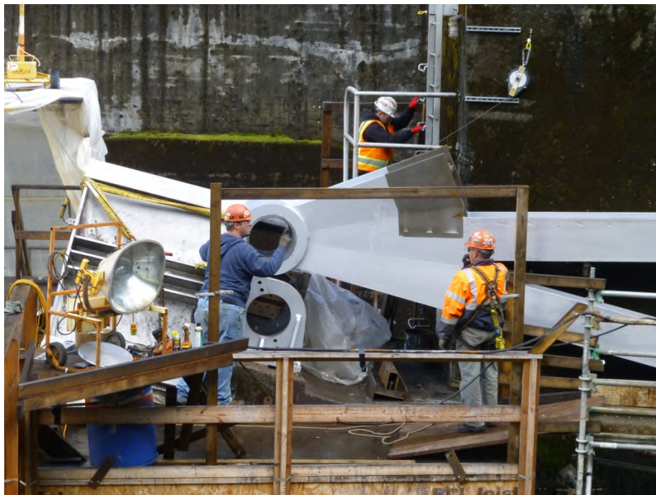
Figure 12-25. Spillway Tainter Gate Trunnion Bushings.
