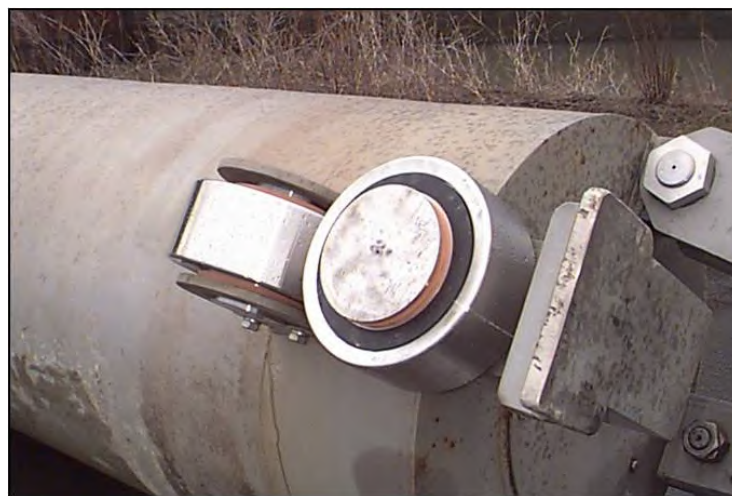
Figure 12-23. Floating Mooring Bit Self-Lubricated Guide Rollers.
