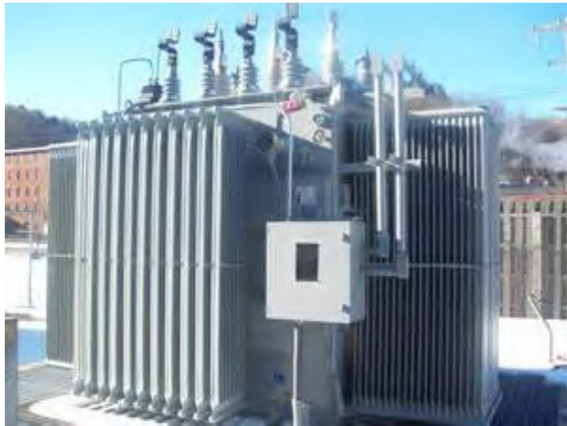
Figure 13-2. Transformer at a Power Plant.
