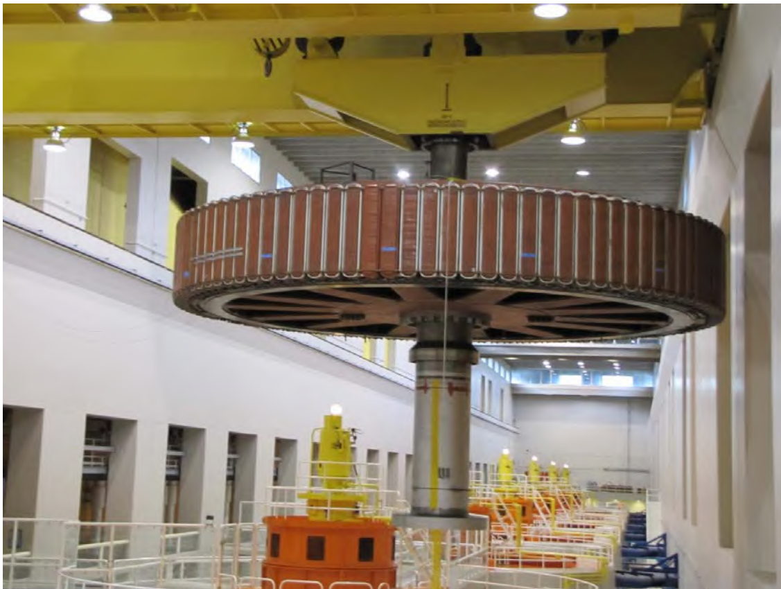
Figure 9-7. Generator Rotor (460-ton).
