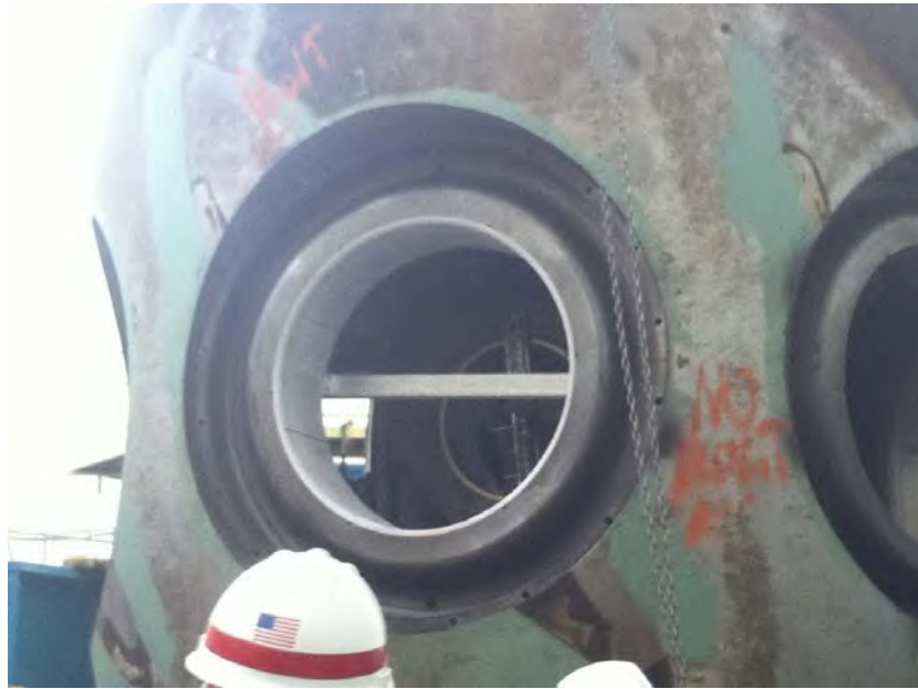
Figure 12-33. Kaplan Turbine Hub Bushings.
