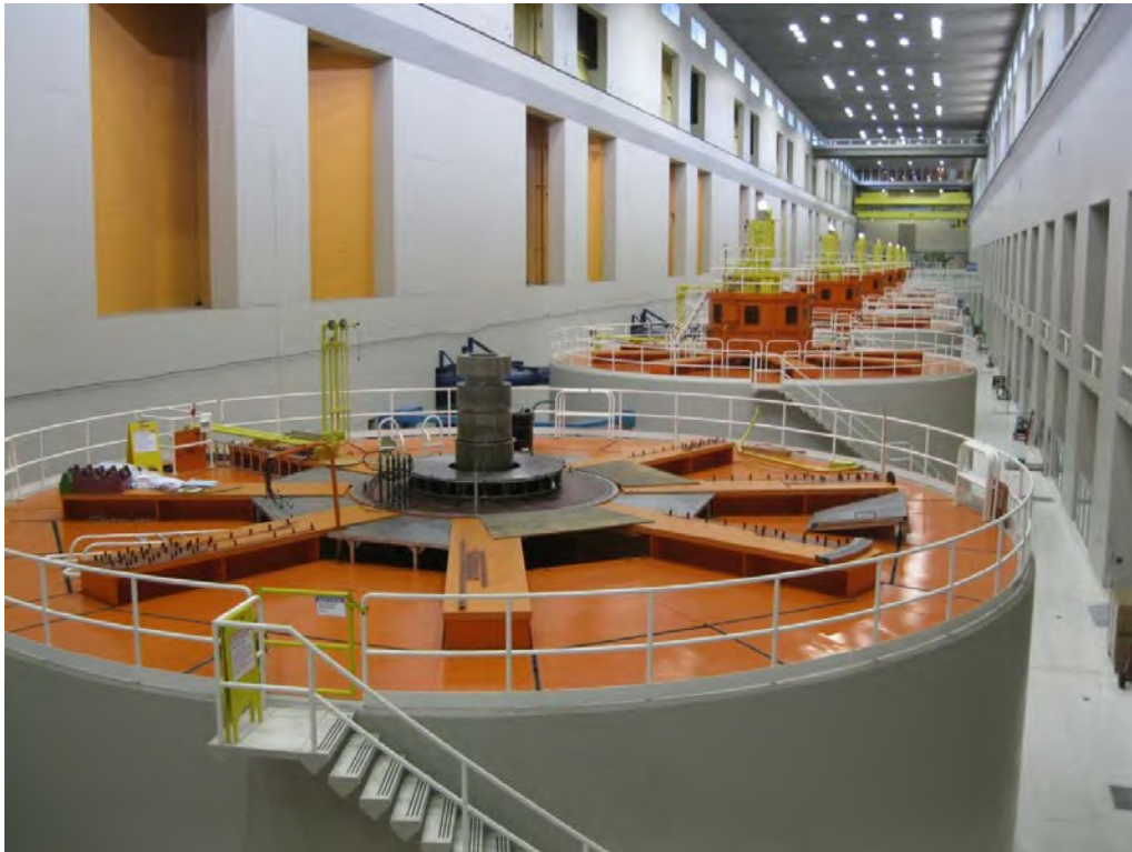
Figure 9-1. Bonneville Dam – Hydroturbine Units.
